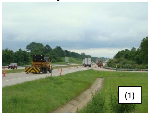
Picture 1 shows an acceptable exit ramp closure.
