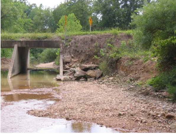
(1) Indian Creek -- Howell County Roadway Embankment Scour Upstream End
