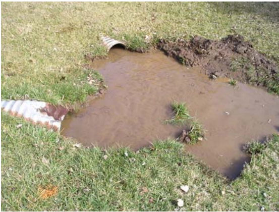
(1) Downstream Culvert Ditch (Silted In)
