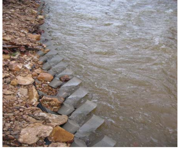
(8) Ajax Blocks Performing Under Full Flow Conditions
