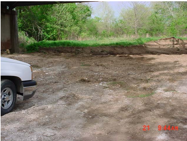
(9) Erosion under structure
