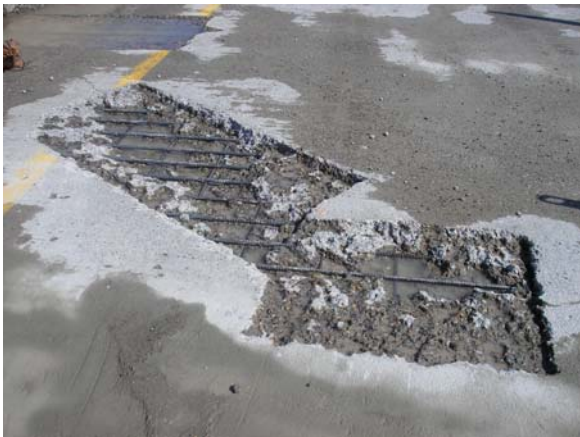
(5) Close Up Showing Exposed Rebar
