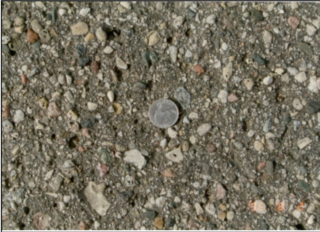
Figure 4.11. Example of a badly pocked, porous and oxidized surface.
