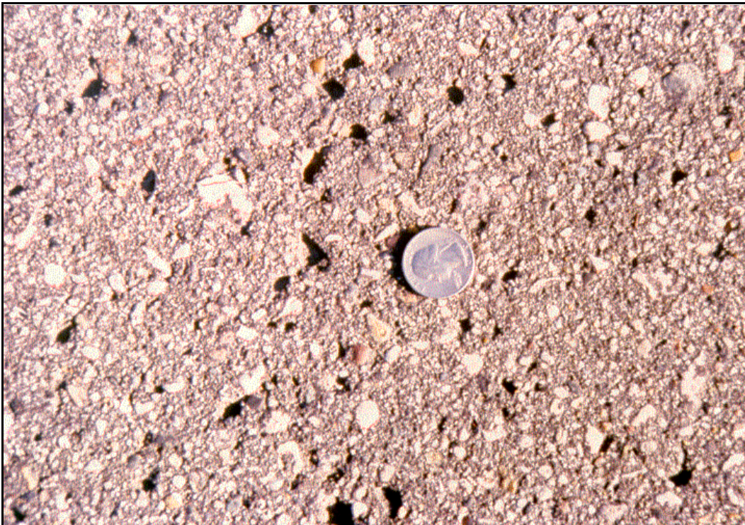
Figure 4.10. Example of a slight pocked, porous and oxidized surface.
