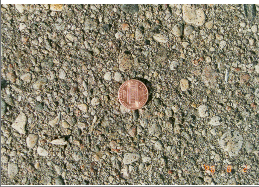
Figure 4.9. Example of a slightly porous and oxidized surface.
