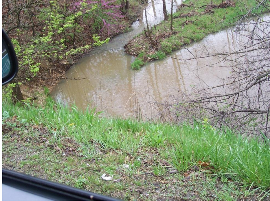
Figure 6.9 Steep dropoff at creek crossing (Rossy et al., 2009).
