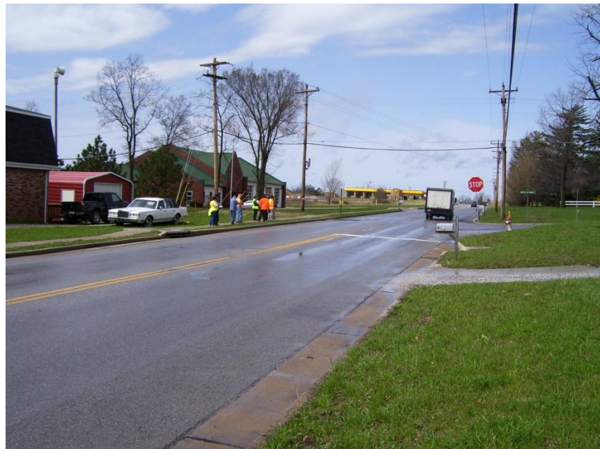
Figure 6.11 Pavement rutting on St. Charles Road (Rossy et al., 2009).
